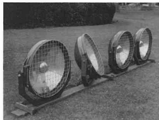
Set well back from the building, low-surface brightness projectors are used to light most of the main fabric of the Cathedral.
