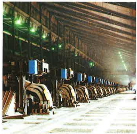
Aluminium production in an electrolysis shop
