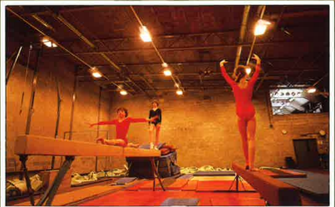
WE'RE CONSERVING OUR ENERGY AT BANGOR 250W SON Deluxe lamps illuminate the gymnasium at Bangor University, North Wales.
