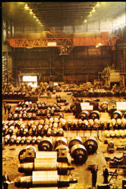
The first 1000W. Solarcolour installation in Britain at Llanwern BSC Roll Shop; brought increased illuminance and saved power.
